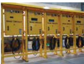
Battery Charging Station
